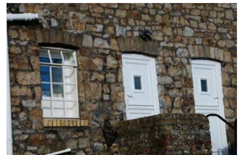
Traditional steel window which is appropriate adjacent to new white uPVC doors that are not. Note also inappropriate white uPVC pipework.
