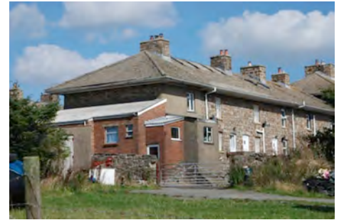
Insensitive extensions to the prominent west end elevation of Lower Row.
