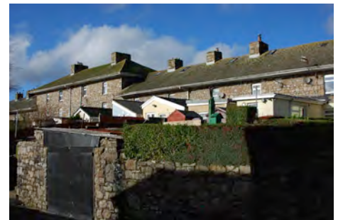
The rear of Collins Row with an eclectic mix of shoot-out extensions with differing roof forms that do not complement the designed and unified nature of the rows.
