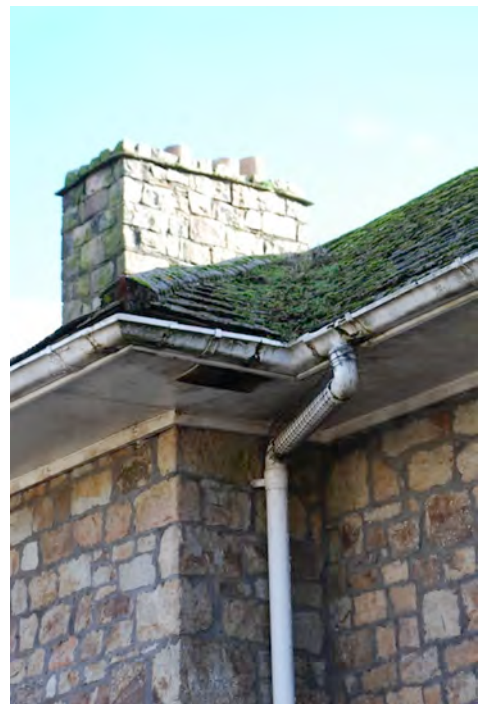
Detail of existing roof / eaves arrangement. The existing tiles attract excessive moss growth. The plain soffit and large diameter downpipes are inappropriate details in the context of Bute Town's heritage.
